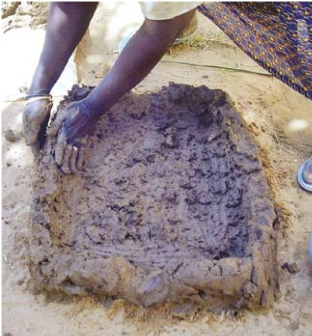
Pic 73. The exhaust hole is cut out of the end of the stove.
