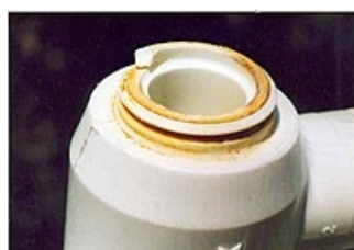
Chlorine attack of acetal resin plumbing joint
