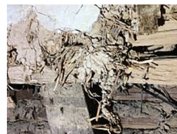
Lime setting-coat on clay plaster with straw binder. Applied to hand-split lath over a timber framed wall of a brick family house at Economy Landmark village.
