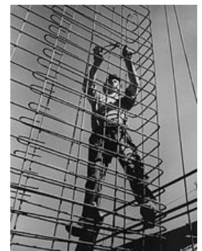
Constructing a rebar cage that will be permanently embedded in a finished reinforced concrete structure
