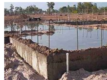
A concrete slab being kept hydrated during water curing by submersion (ponding)
