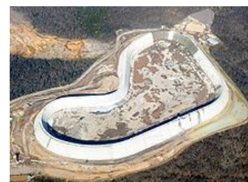
Aerial photo of reconstruction at Taum Sauk (Missouri) pumped storage facility in late November, 2009. After the original reservoir failed, the new reservoir was made of roller-compacted concrete.
