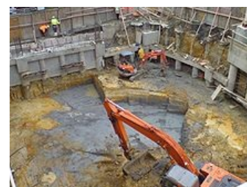
Clay layers in a construction site. Dry clay is normally much more stable than sand with regard to excavations.
